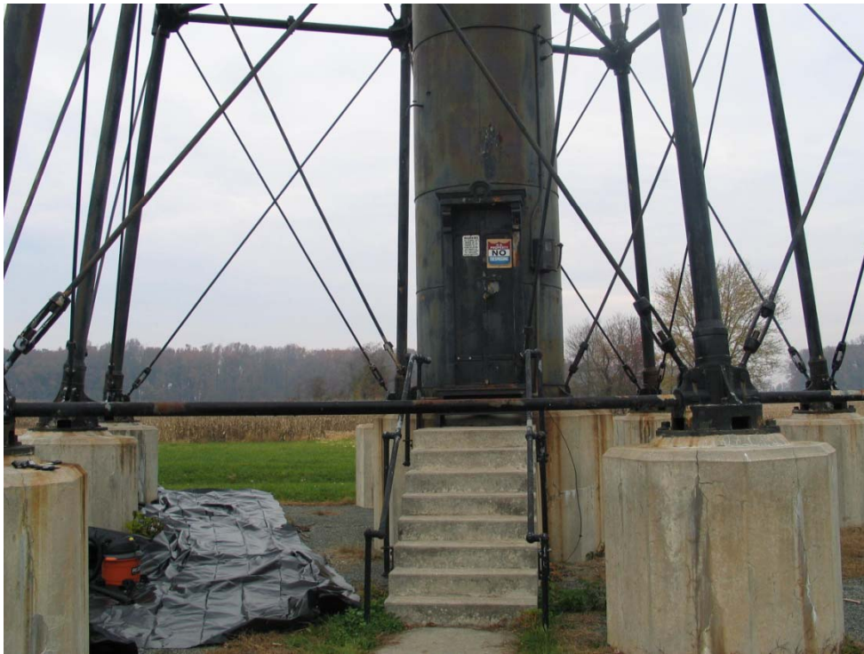
Initial site conditions. Note plastic sheeting being placed prior to lead based paint removal.
