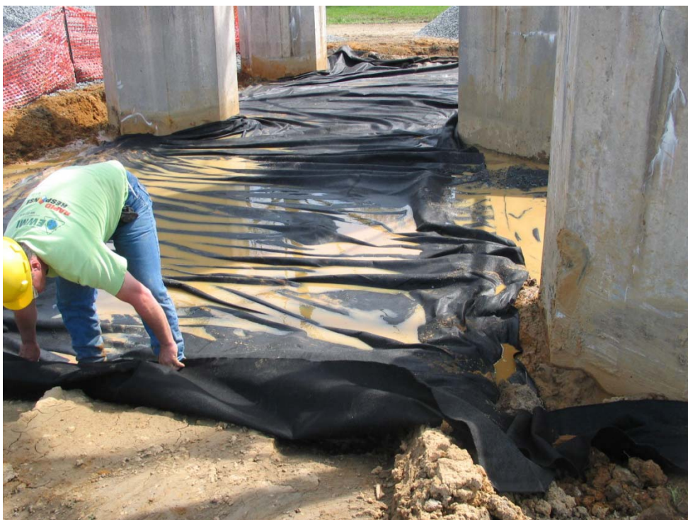
Installation of filter fabric above excavation floor to support the stone to be used as backfill.
