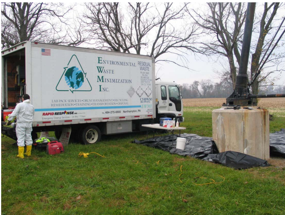
Crew preparing Level C PPE for lead based paint removal. Decontamination station over plastic sheeting.
