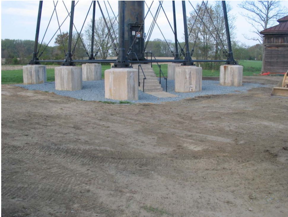
Excavation completely backfilled; subbase of the site has been regraded prior to restoration.
