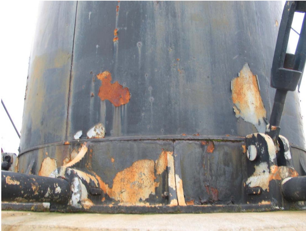
Typical condition of existing paint.
