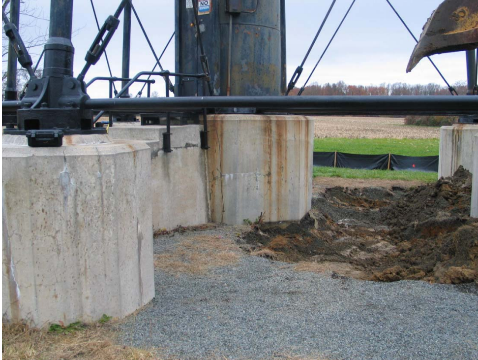
Note repainted cross brace and joints (left side) and initiation of excavation.
